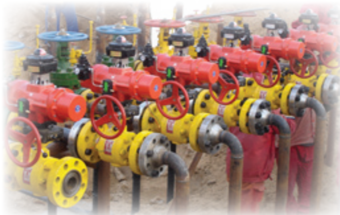
Conducciones de gas (China) Oilfield gas conductions (China)
